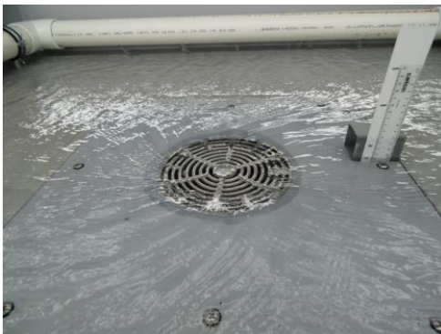
Weir Flow – 2.5 L/s (20mm)
